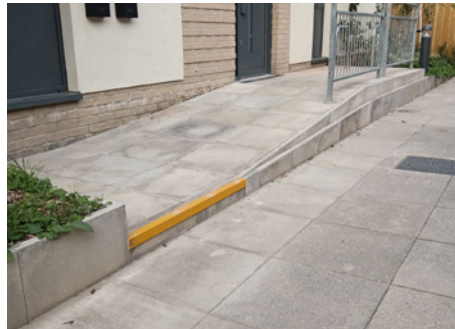
Above: The ramp at Great Barn Court ends in a step. Image: Tracie-Jane Bath. Right: Council cabinet member for housing Matt McCabe
